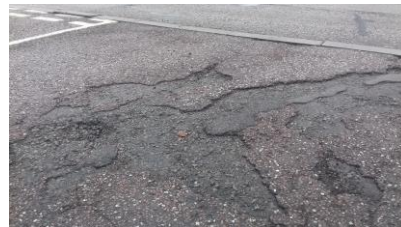
Above: Damaged road below intervention. Saxon Gate Church Of The Cornerstone.
