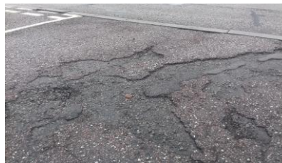
Above: Damaged road Saxon Gate.
