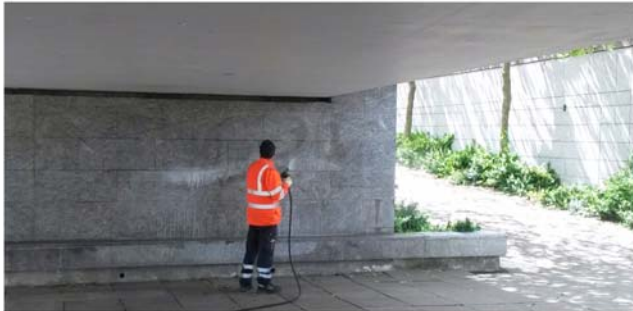
Above: Before and after; graffiti at Campbell Park underpass.
