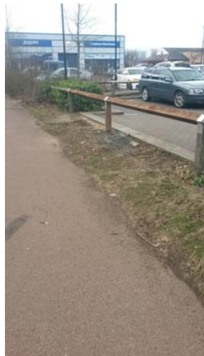
Above left: Criminal damage to posts near Cotswold.
