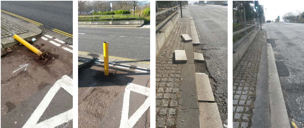
Left: Broken bollard at Bankfield Roundabout. Second left: Bollard fixed at Bankfield Roundabout. Third left: Potholes and misplaced paving at Witan Gate near Law Courts. Right: Replaced paving and filled potholes at Witan Gate, near Law Courts.
